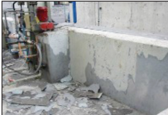
Failed coating after spills
